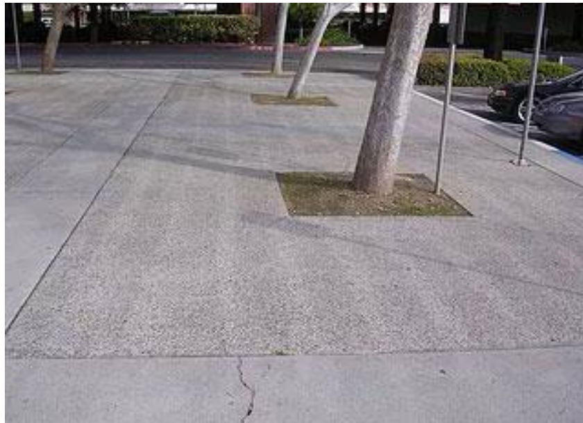
*Streaks from uneven washing and improper pre-treatment of surface
