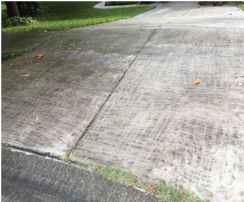
*Scratching and incomplete washing due to improper equipment (wand vs surface washer)
