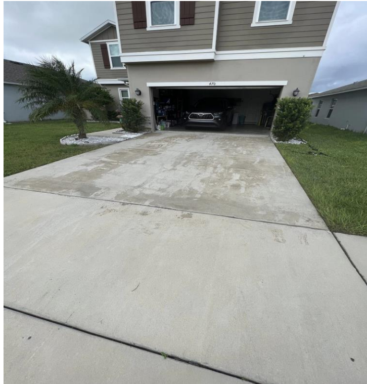
*Acid Stains on Driveway from improper use of chemicals.
